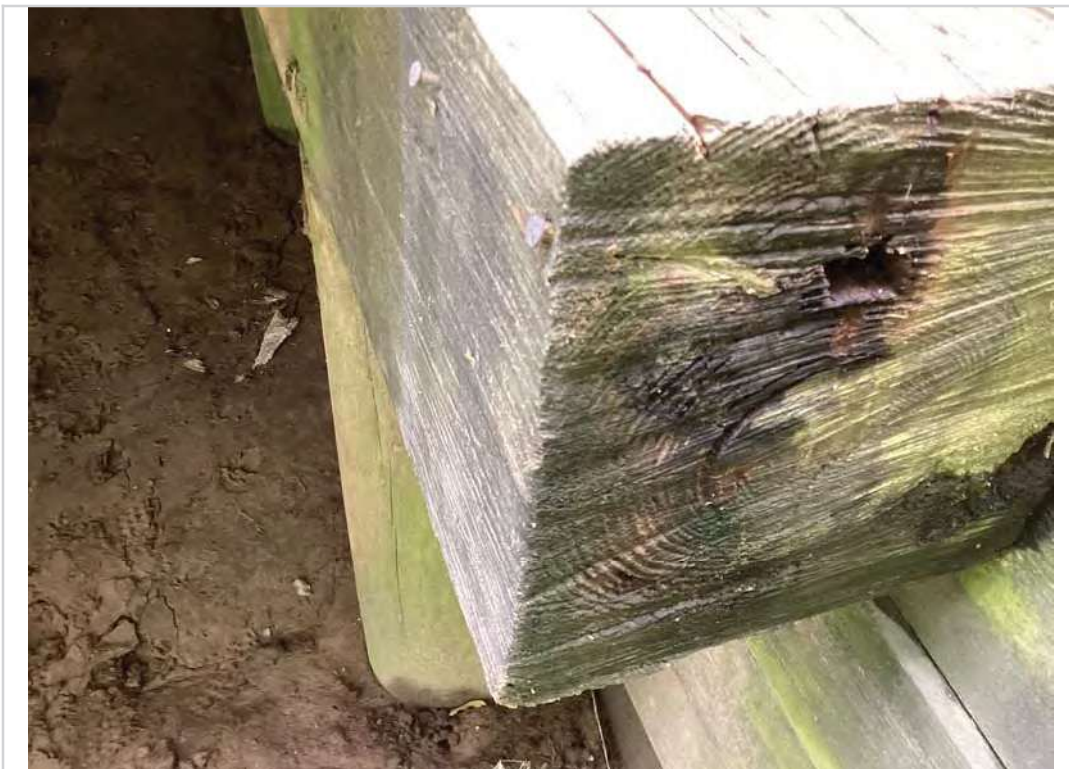
Abutment 1 left end decay area
