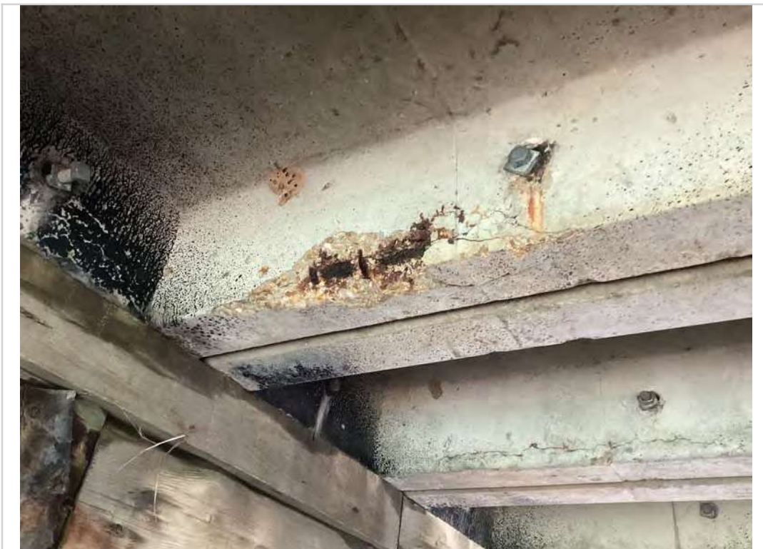
Spall to steel slab C span 2
