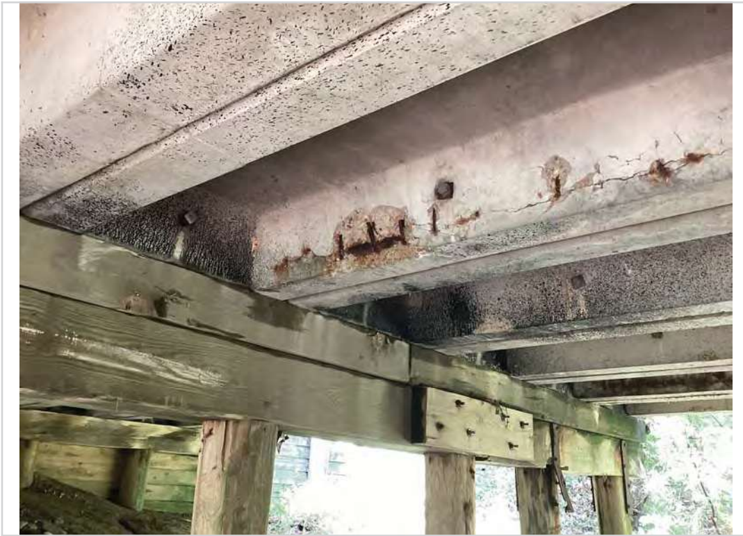
Spall to steel slab E span 2
