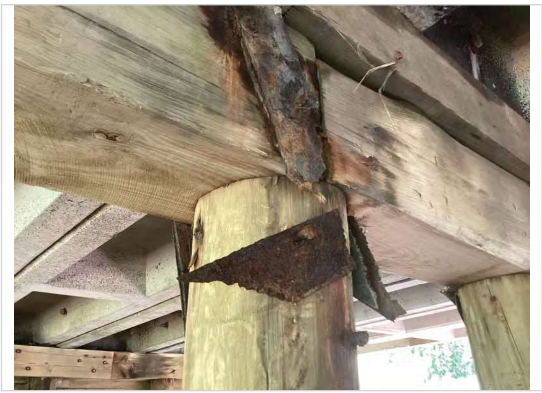
Bent 2 grader blade rusted in half
