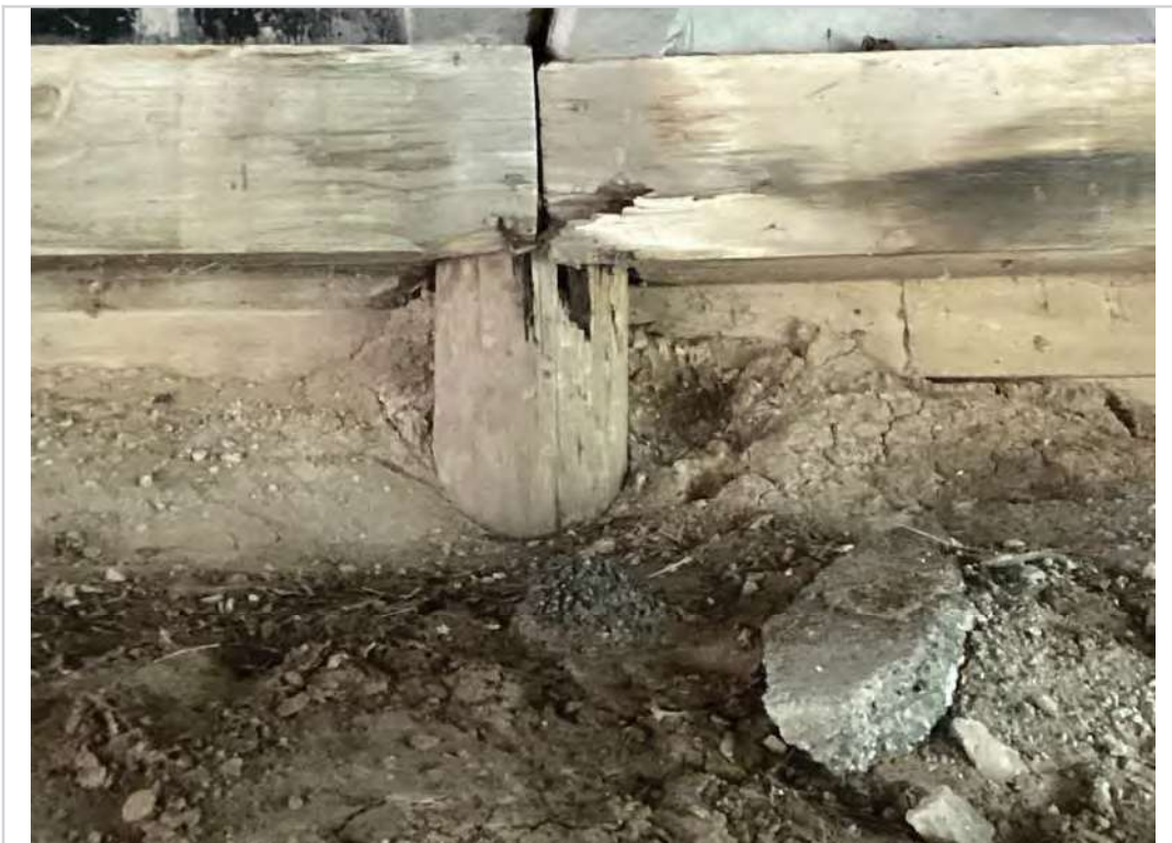
Abutment 1 pile D decay area. Cap above pile D decay area
